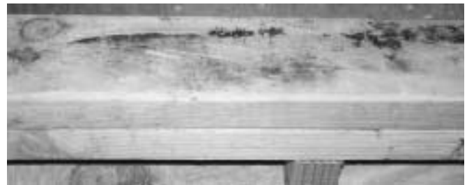
Fig. 3: Mold on lumber
